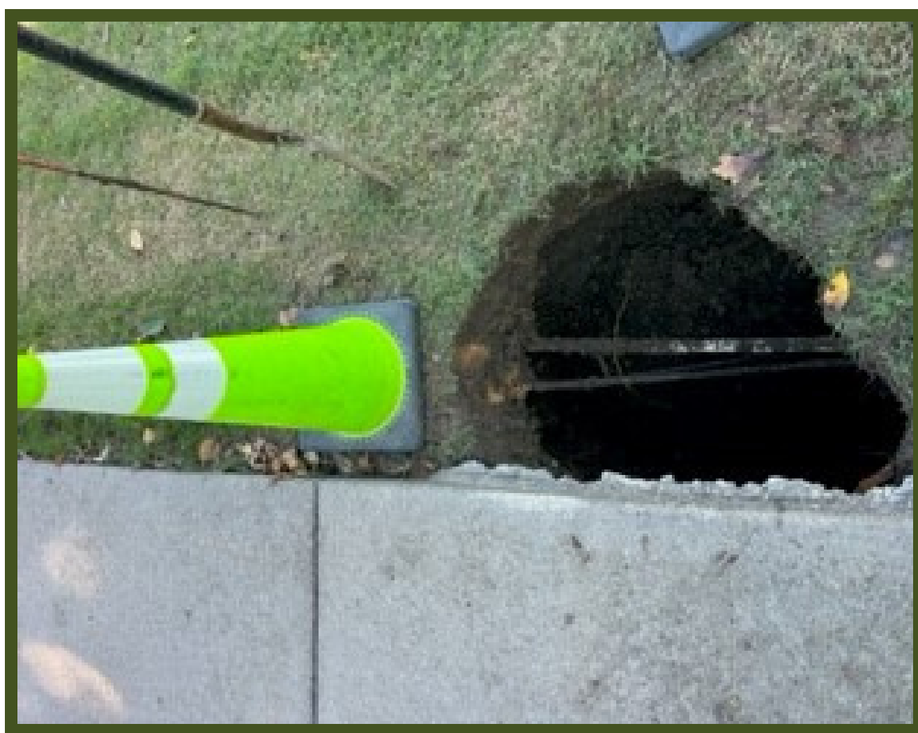
EMERALD BAY SINK HOLE REPAIR BEFORE
